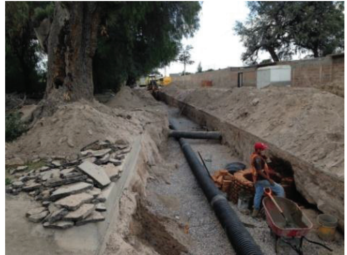
SUBCOLECTOR SANITARIO ZAMARRIPA
